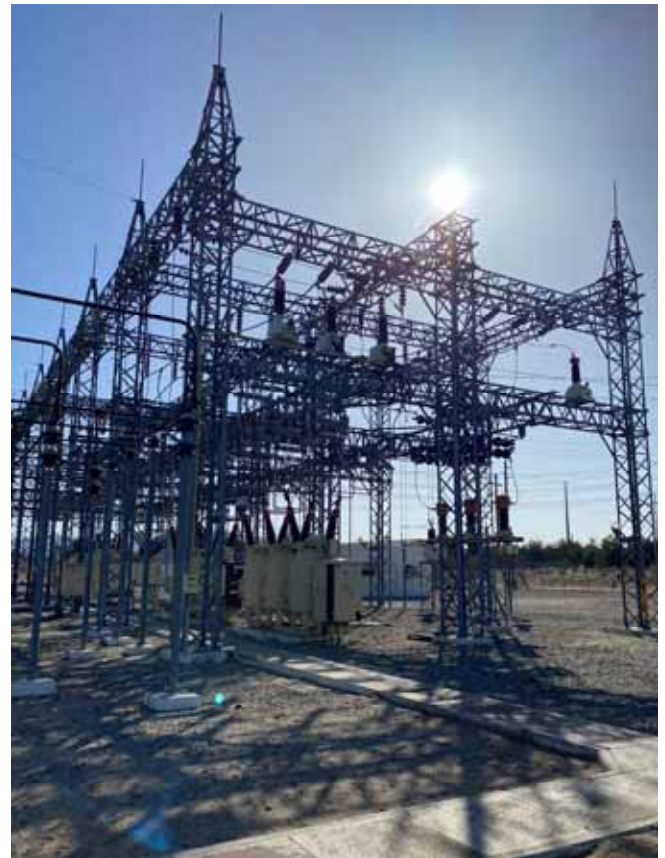
Figure 18. South facing view of Gila 34.5-kV yard
