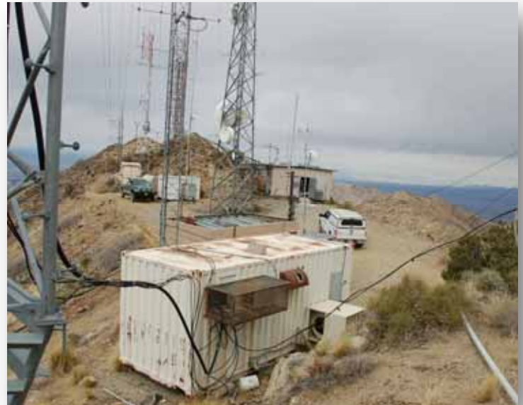
Figure 7. Crossman Peak Microwave Facility
