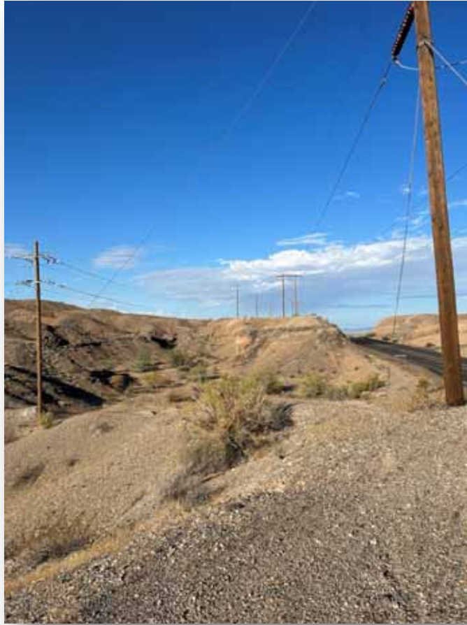
Figure 15. WAPA tie-in to the PAD-HDR line looking south
