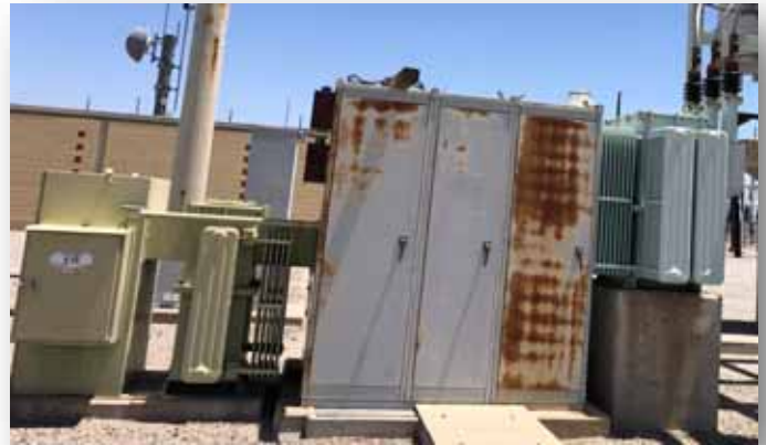
Figure 5. Liberty Substation Station Service Equipment
