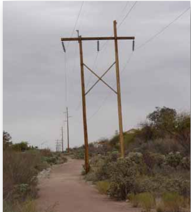
Figure 9. Oracle-Tucson H-frame and single pole structure
