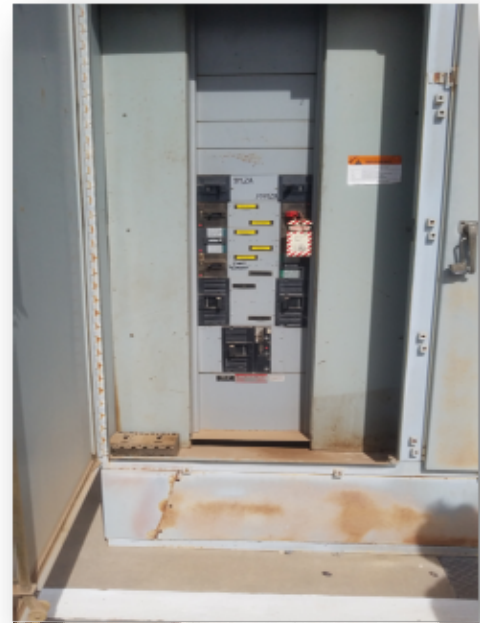
Figure 10. Coolidge Substation Distribution Panel
