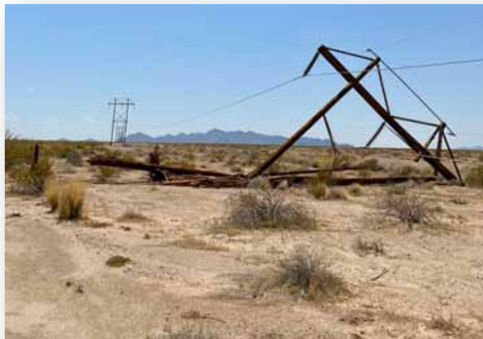
Figure 16. PAD-BLY#2 structure 25/7 damaged July 2024
