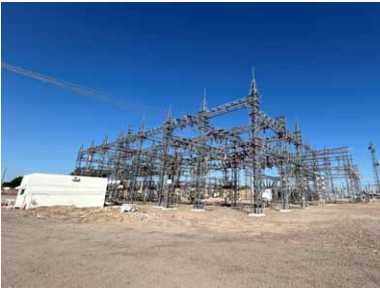
Figure 17. Northeast facing view of Gila 34.5-kV yard
