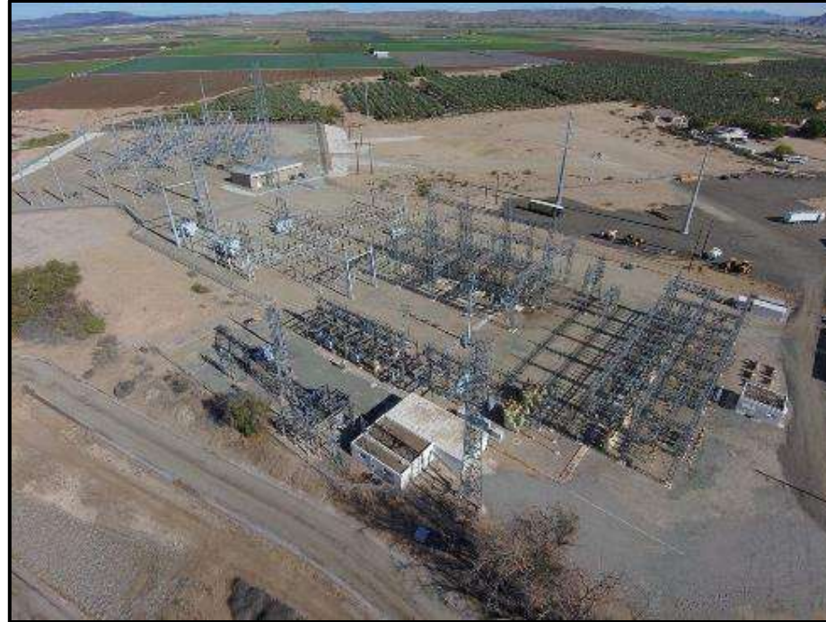
East view of Gila Substation
