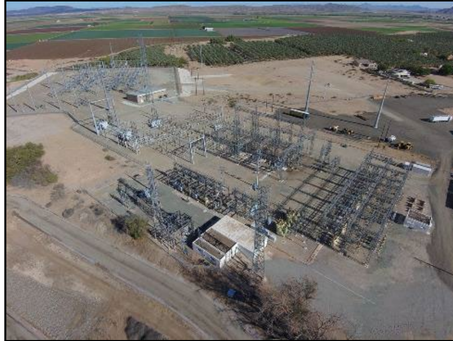
East view of Gila Substation
