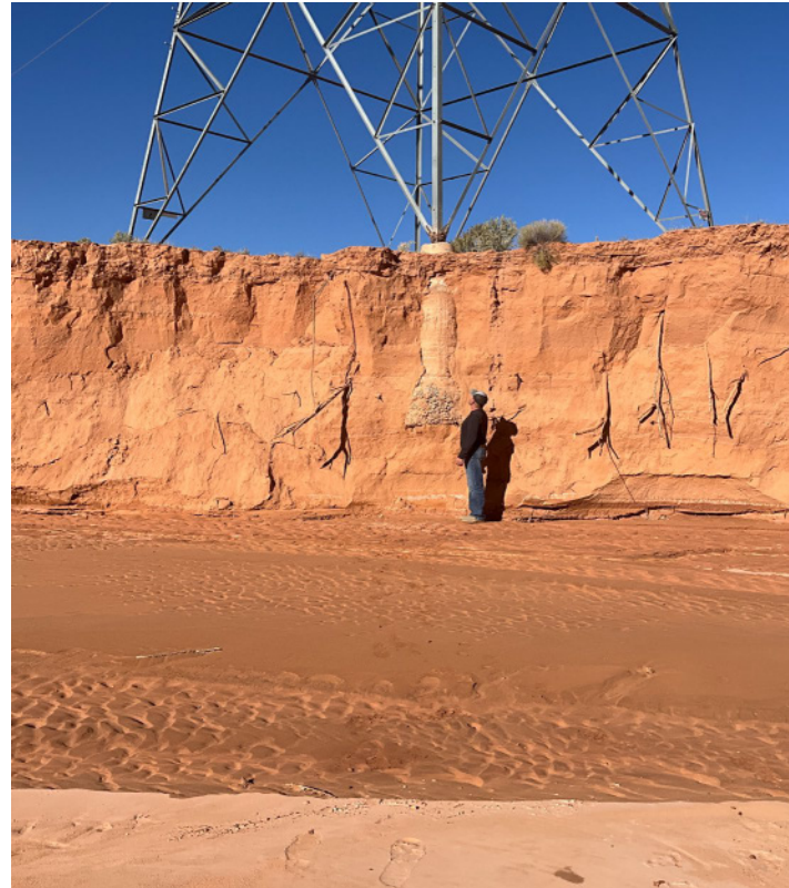
Tower 77-1 in October 2025, footing became exposed
