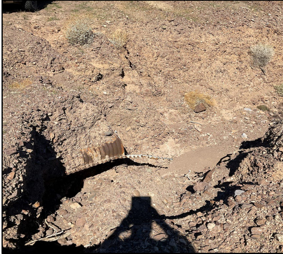
Deteriorated and washed-out culvert
