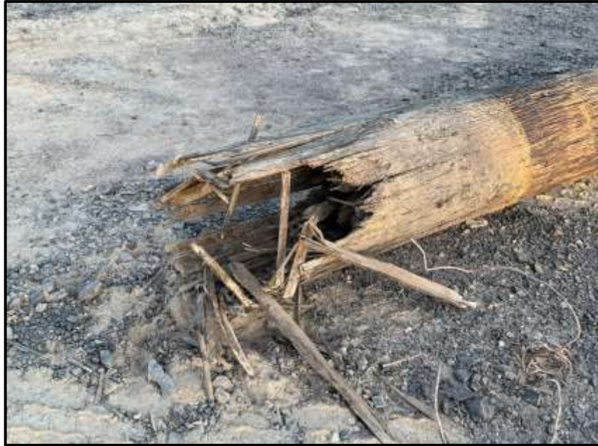
Severe pole rot visible after removal
