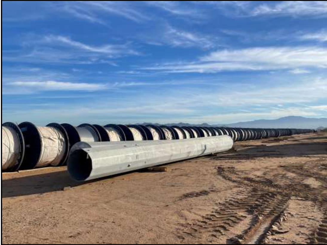
Conductor and Steel at Avra Valley Laydown Yard
