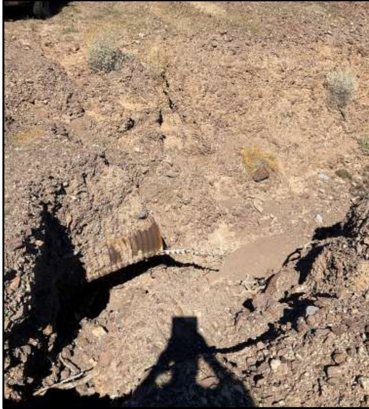
Deteriorated and washed-out culvert
