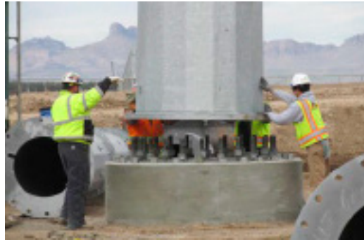
Construction crews secure the next section of the Saguaro line structure that is part of the ED5 substation upgrade.
