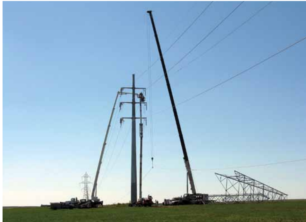
Above: A steel monopole is erected to replace the existing steel lattice structure, Aug. 20, on the Fort Thompson-to-Huron 230-kilovolt double-circuit line. With the appropriate ground clearance, the line can now be operated at maximum capability safely and reliably. UGP has been modifying several spans to ensure appropriate ground clearances since 2011, including replacing towers, excavating ground and raising existing towers. (Photo by Joel Miller)
