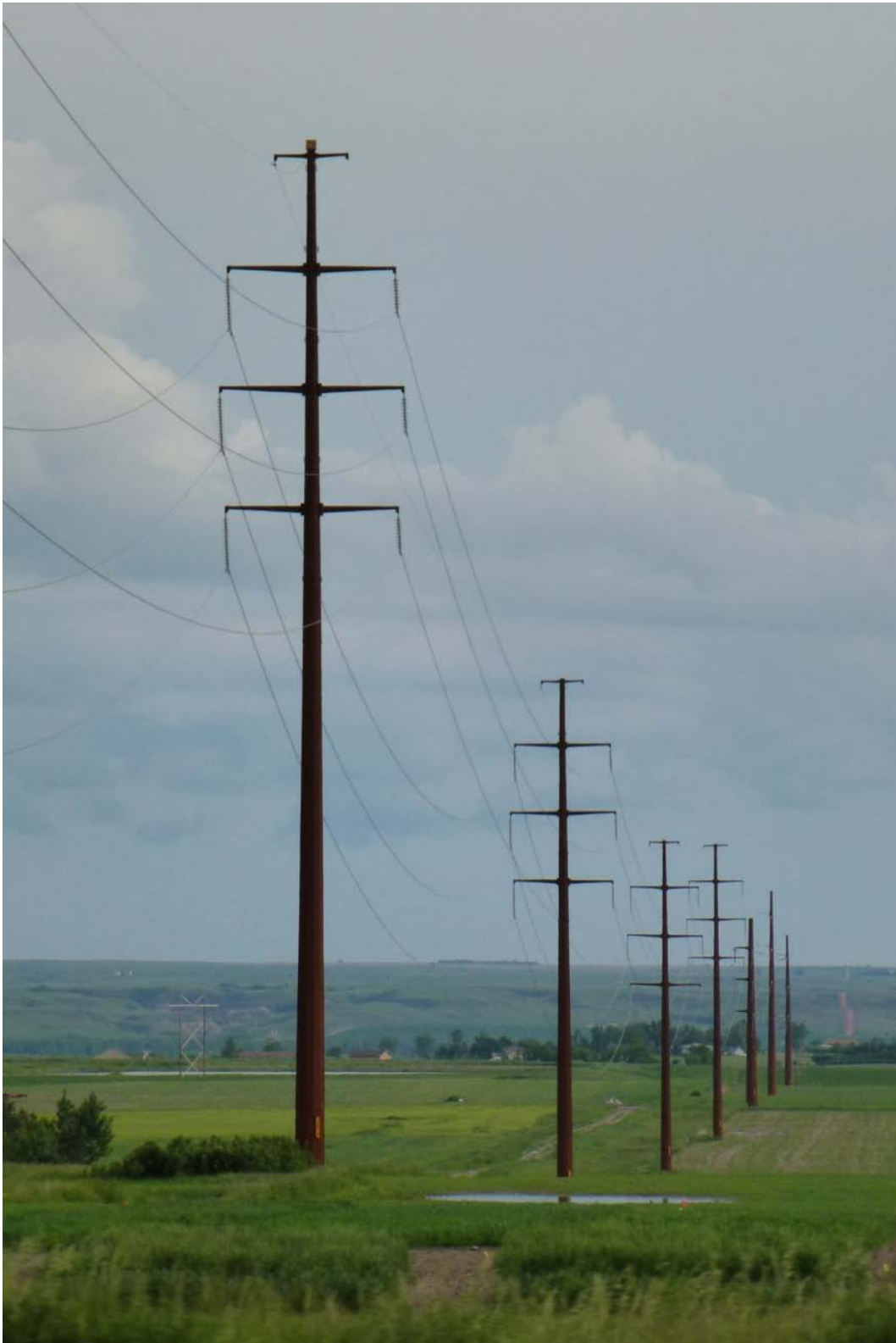
Figure 2.3-3 Single Pole Double circuit 230/115-kV Structure
