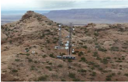
APS tower site at Jack's Peak
