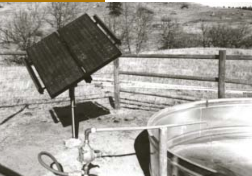
Photovoltaic installations often make financial sense at remote locations, such as this stock watering tank. Building a power line to serve an isolated load is not typically cost-effective.
