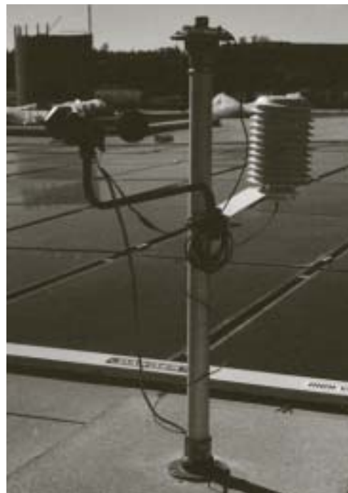
Rooftop photovoltaic installations like this one at the Elverta Operations Center demonstrate Western’s interest in renewable energy technologies.
