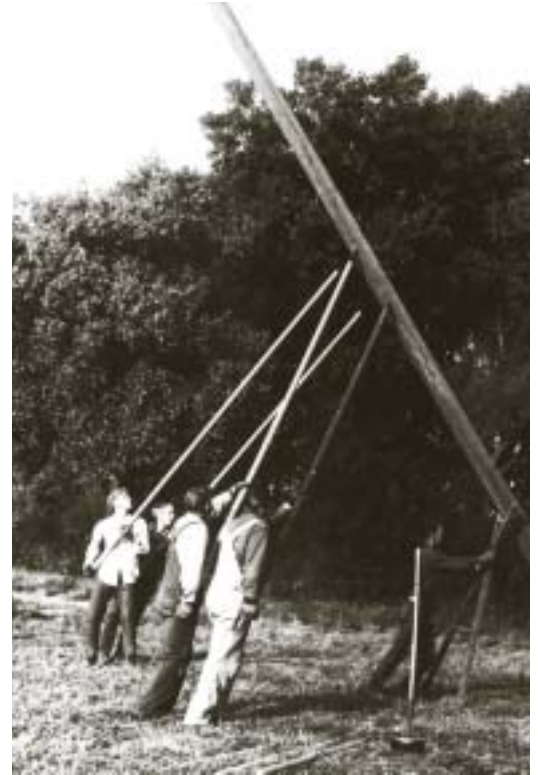
By the time of the California-Oregon Transmission Project, construction techniques had advanced from hand-powered pole raising (above) to helicopter-aided construction techniques (below).
