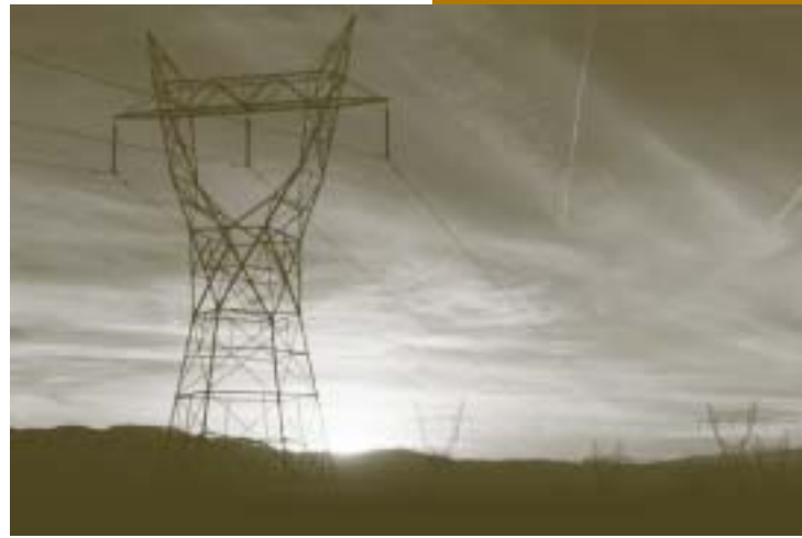
Transmission lines are the electron highways that carry electricity from the generating facility to the utility.
