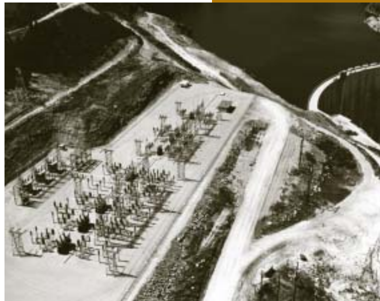
Switchyards connect the transmission grid with generating plants. (Photo by the Bureau of Reclamation)
